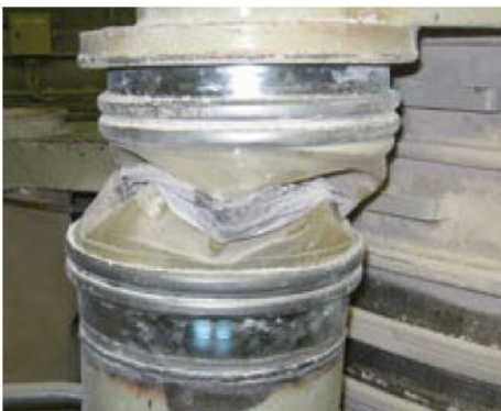
INSTALLATION GAP TOO SHORT
